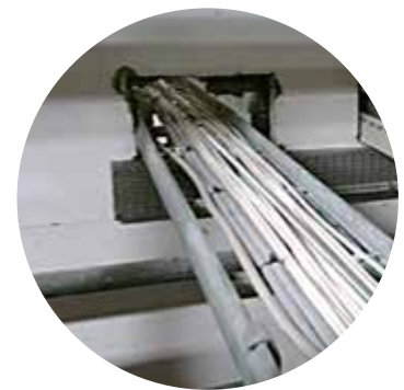
Picture shows an example of unsealed penetrations through a fire rated wall.
