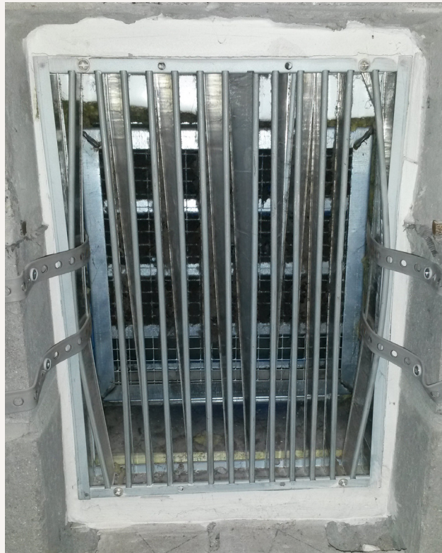
An example of the incorrect installation of intumescent dampers.
