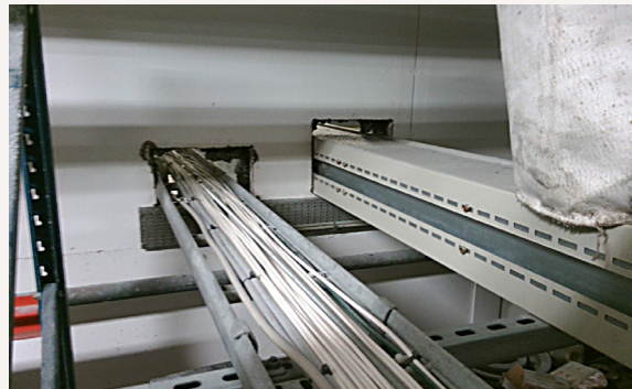
Picture shows an example of unsealed penetrations through a fire rated wall.
